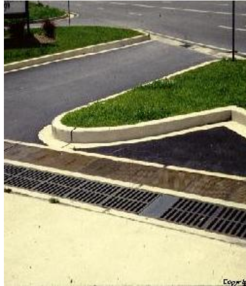
Figure PTP-01- 6 Perimeter Sand Filter
