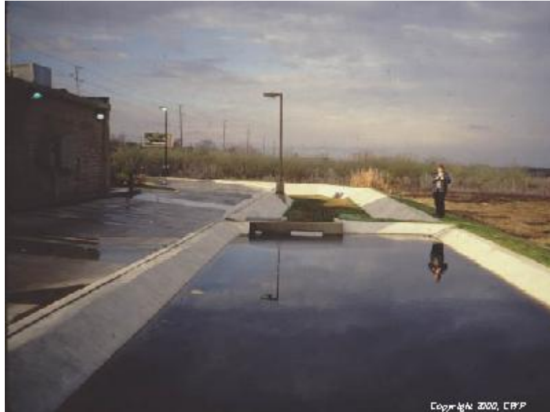
Figure PTP-01- 2 Surface Sand Filter
